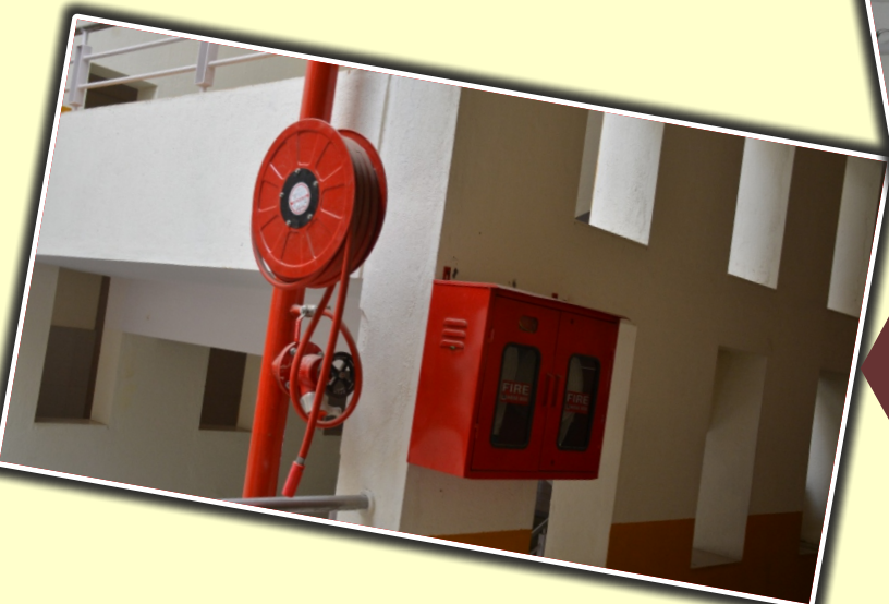
Fire Fighting System
